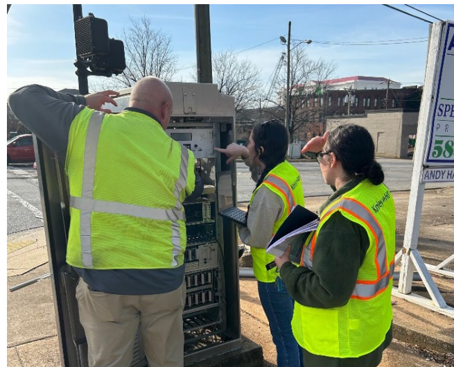
Traffic Signal Timing Implementation
